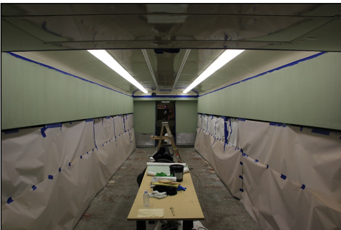
A view of the new wall finish inside the diner. This is in close approximation of the look the IC had in the car, as we were unable to match the original material for a reasonable cost.
