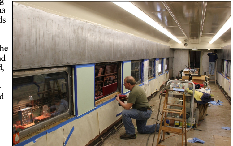
John Bratcher is drilling holes for window re-tainer, while in the background Tylene Crouch is stripping old wallpaper adhesive.
