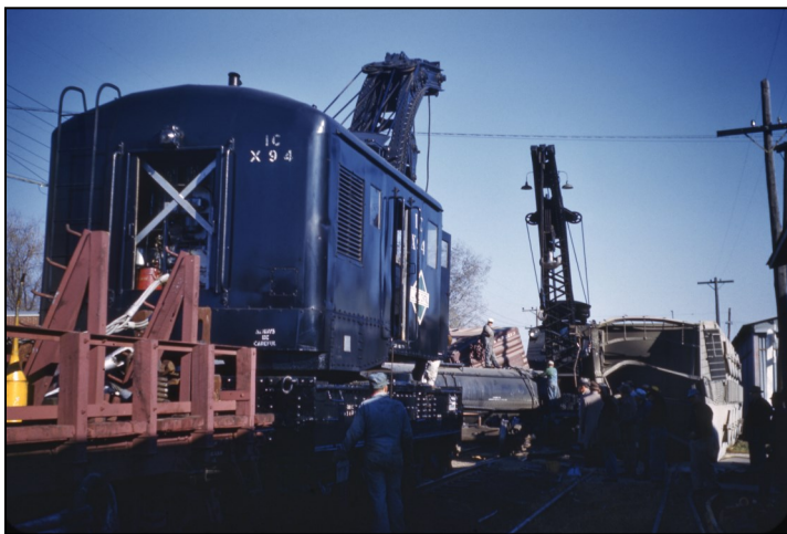
IC derrick X94 works at the western end of the derailment near Hamilton Street. This photo is looking east from what is now the platform of the Museum’s Wabash Depot.
