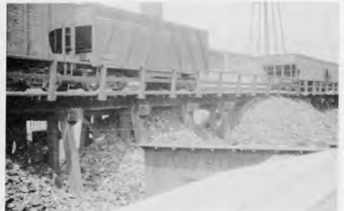
Timber Coal trestle for Malleable Iron Works. 2 miles N. of Rockford - 537' long, built 1907.
